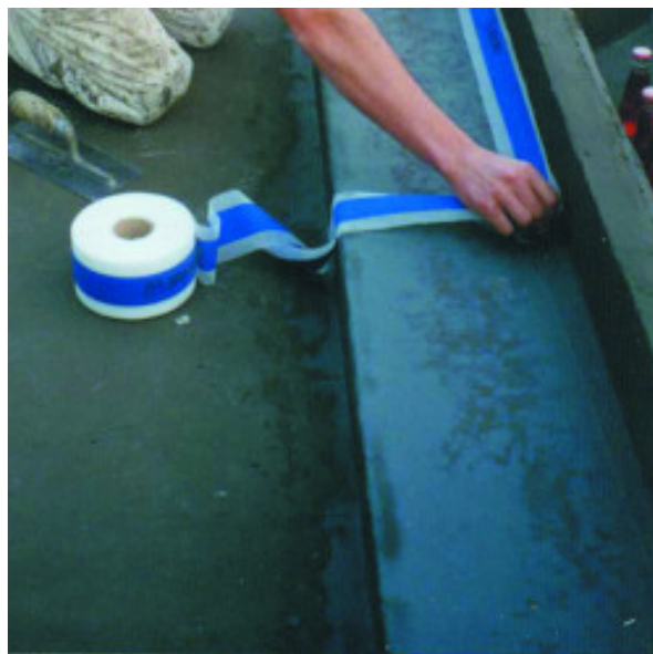
An example of Mapeband waterproofing a corner between the bottom and a side of a bath tub
